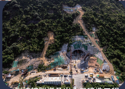
副連接隧道及出入口建造工程 Construction of Secondary Access Tunnel and Portal
