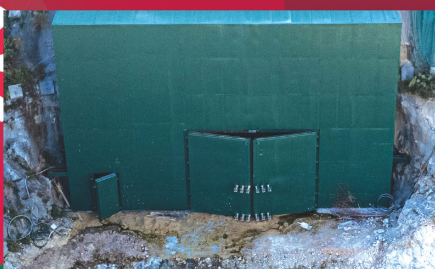
副連接隧道的防爆門 Blast Door for Secondary Access Tunnel
