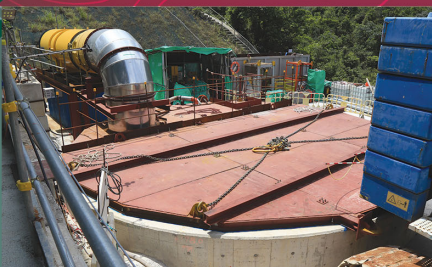
通風井防爆罩 Blast Cover for Ventilation Shaft
