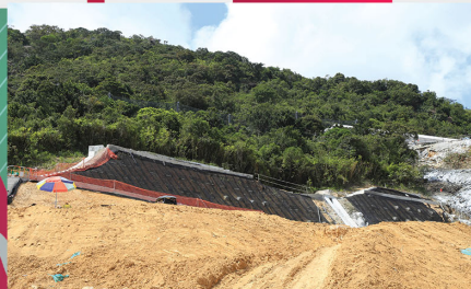
副連接隧道口的斜坡鞏固工程 Slope Stabilization Works above Secondary Access Tunnel and Portal
