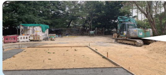
社區聯絡中心地盤平整 Site Formation Works of Community Liaison Centre (CLC)
