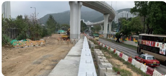
亞公角街隔音屏地基工程 Footing of Noise Barrier along A Kung Kok Street
