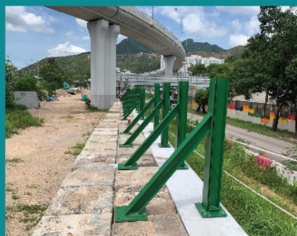
亞公角街臨時隔音屏建造工程 Construction of Temporary Noise Barrier along A Kung Kok Street.
