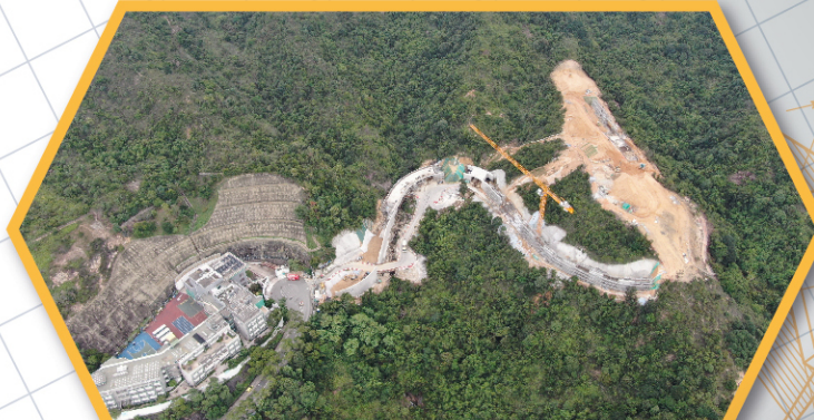
建造連接通風井的道路 Construction of Access Road to Proposed Ventilation Shaft
