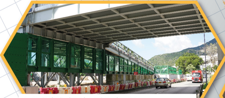
亞公角街臨時隔音屏障建造工程 Construction of Temporary Noise Barriers along A Kung Kok Street
