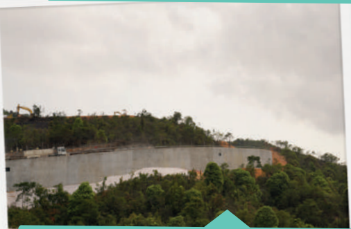
連接通風井道路擋土牆建造工程 Construction of Retaining Wall along the Access Road to Ventilation Shaft
