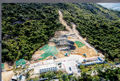
副連接隧道及出入口建造工程 Construction of Secondary Access Tunnel and Portal
